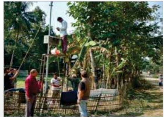
Solar Street lights in village Barsimaluguri village, Assam
