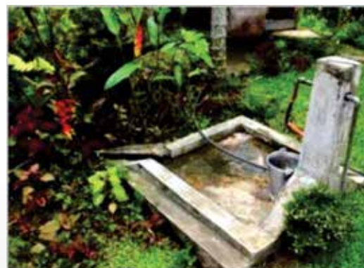
Common water supply connection for 3-4 houses Mawlynnong, Meghalaya
