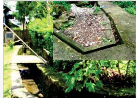
Storm water network along 100% street network Mawlynnong, Meghalaya
